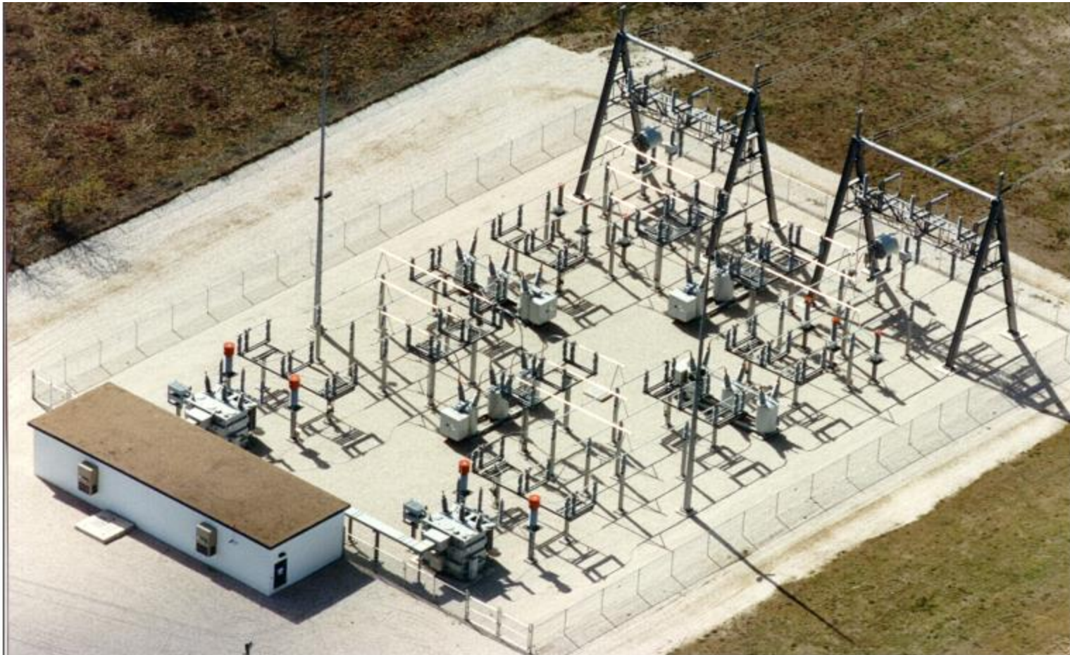
Typical 138 kV Substation
