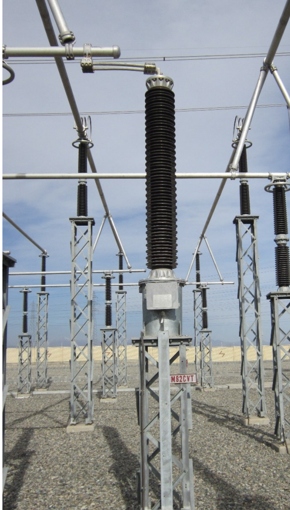
230 kV Bus CVT:
