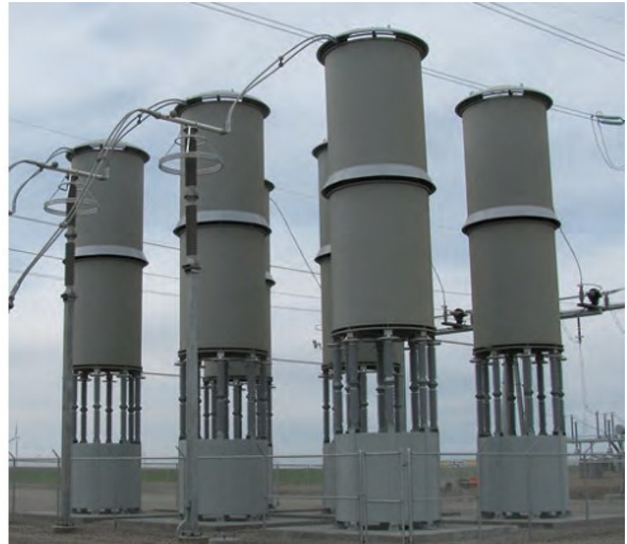
345 kV, 20 Mvar 3-phase shunt reactor
