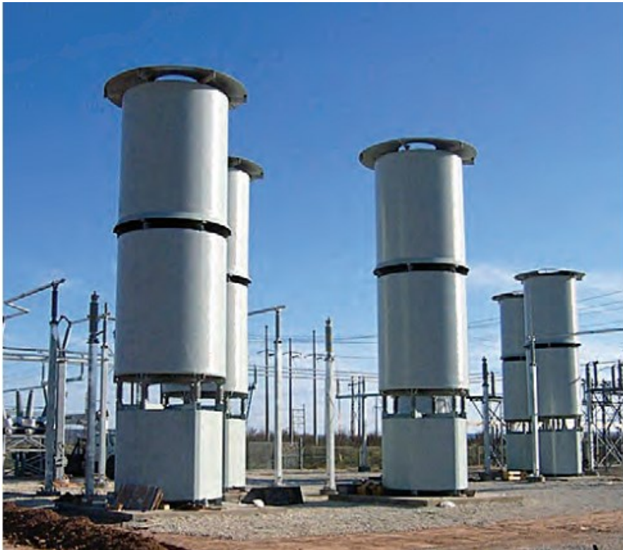
132 kV, 20 Mvar 3-phase shunt reactor (2 banks)
